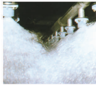
发电厂脱硫塔喷淋
